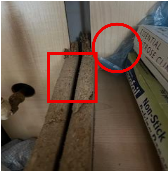
Swelling and cut out pieces may indicate a historic water damage event and likely hidden mould
