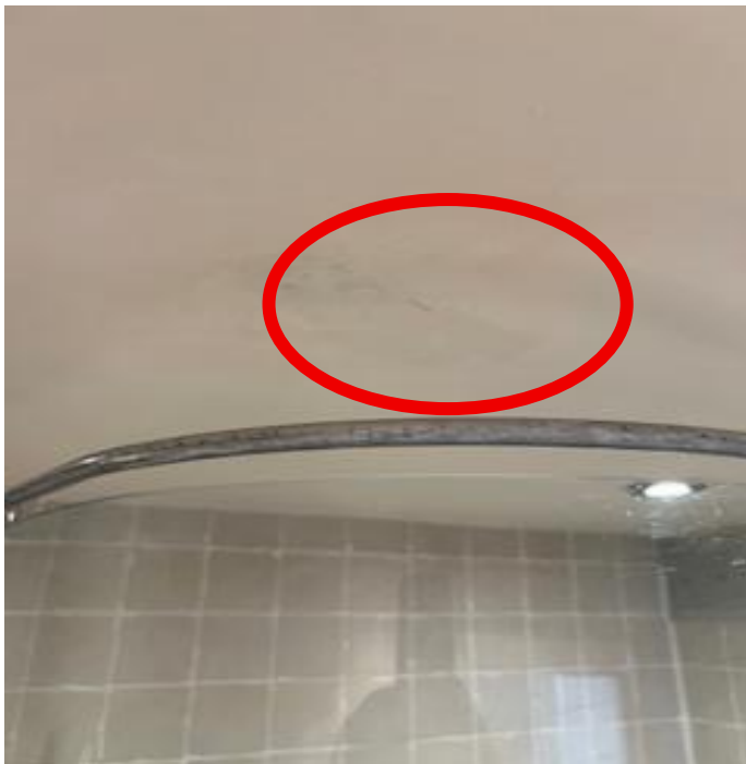
Shower room above, slight staining on a plasterboard ceiling, noted the flat has only two plasterboard ceilings, a shower room and a toilet, the rest is concrete. This is a major concern
