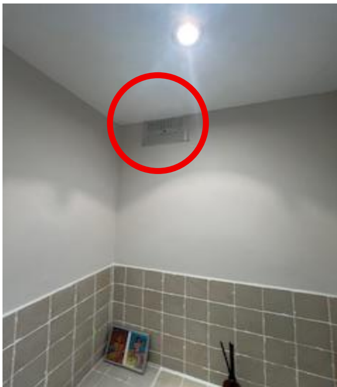
Toilet above, communal extract fan, noted black residue on the surface,
